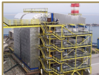
Brindisi Nord Plant
